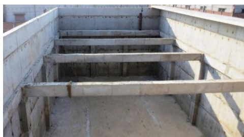
Homogenising Tank before application
