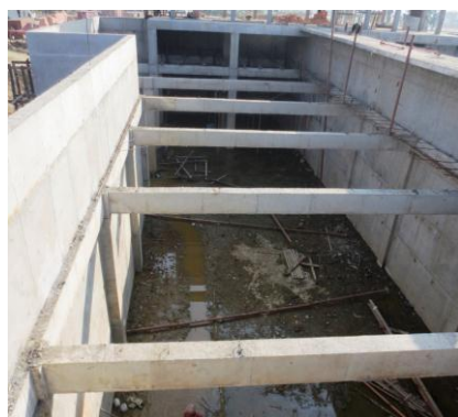
Sedimentation Tank before application
