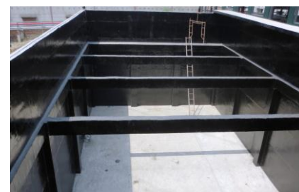
Homogenising Tank after application
